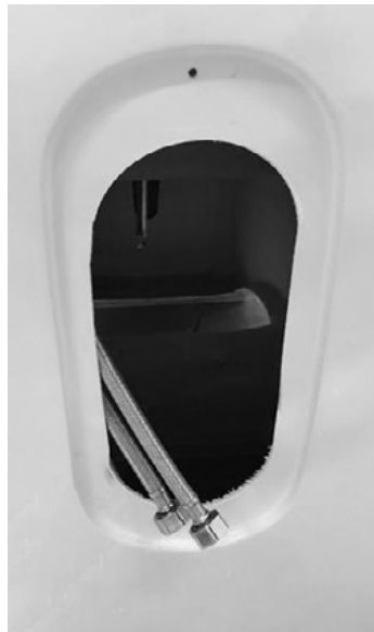
Hot & Cold Water Pipes (back of shampoo chair)
